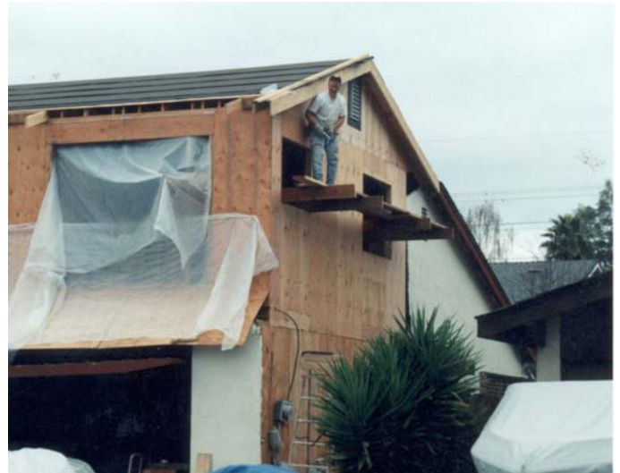
Here I am hanging on by my toenails finishing the sheer wall on the second story.
